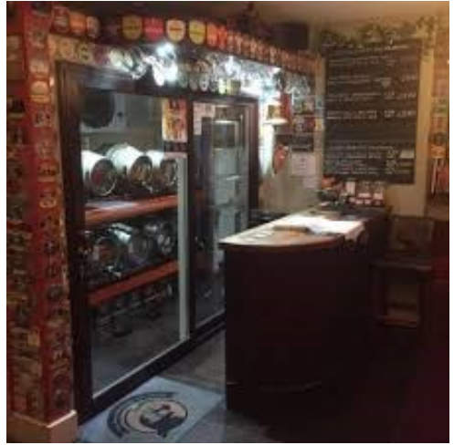
The bespoke chiller room at the Bald Buzzard, Leighton Buzzard
